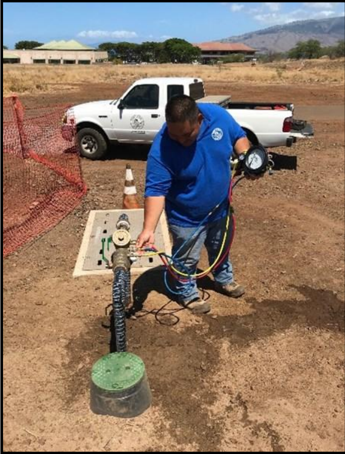
Back Flow Technician Rory Honda testing a newly installed Reduced Pressure Back Flow Preventer at Maui Tech Park in Kihei.
