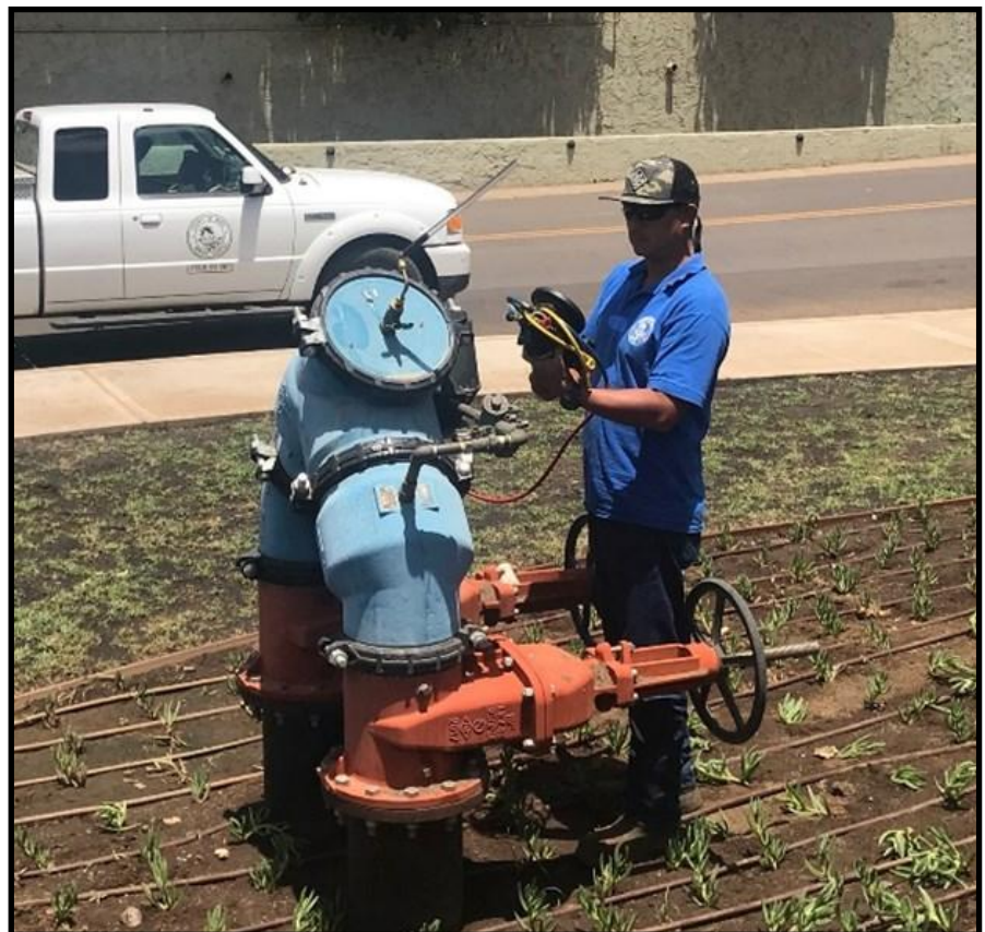
Back Flow Technician Supervisor Kimo Ching testing a new Double Check Detector Assembly at Kalama Kai Condo in Kihei.
